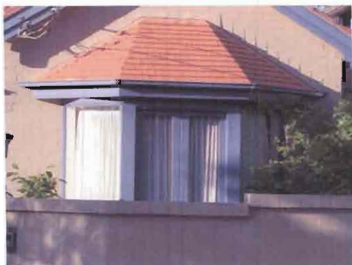
Original joinery has been replaced with new elements that are intrusive and out of character with the dwelling
