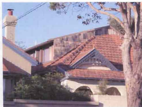
Intrusive Side dormer – siting is appropriate but proportions and materials are intrusive
