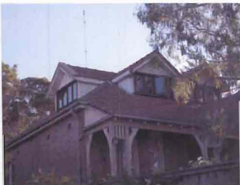
Intrusive Additions- Dormers with poor proportioning and siting, which impacts upon the original roof form to the street
